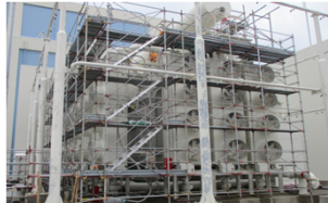
Unit 2 main transformer
