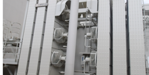
Unit 1 startup transformer
