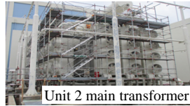
Unit 2 main transformer
