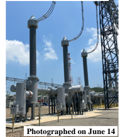
GIS in Naka Noto Sub-station
