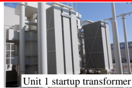
Unit 1 startup transformer
