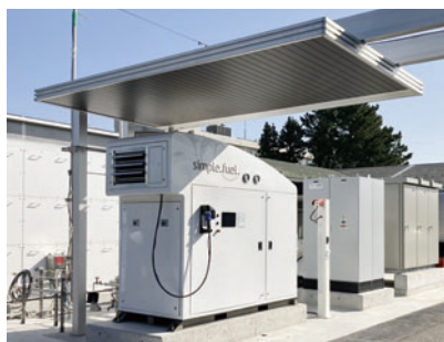
Hydrogen is produced from water at the stations, through electrolysis. (Use of electrolysis powered by renewable-energy-sourced electricity supplied by the Hokuriku Electric Power Company.)
