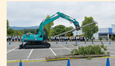
Joint road obstacle elimination drill with local government and the Self-Defense Forces
