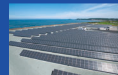
Mikuni Photovoltaic Power Station
