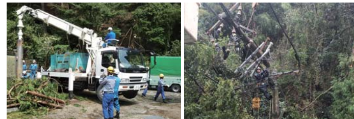
Disposal of fallen trees, removal of damaged equipment, and utility pole construction
