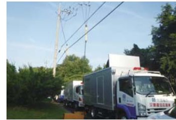
Temporary electricity service with high-voltage power generation vehicles
