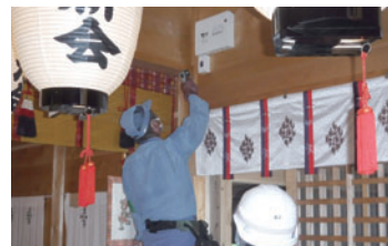
Electrical Inspection of Sumiyoshi Shrine (Tangible Cultural Property Designated by Wajima City)
