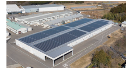
Photovoltaic Panels Installed at a Fukui Byora Co., Ltd. Facility
