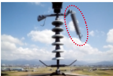
◀ Lightning arrester for transmission
